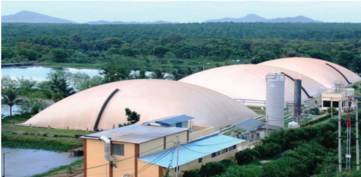
Figure 10. The POME Biogas Plant in Belitung © GIZ
