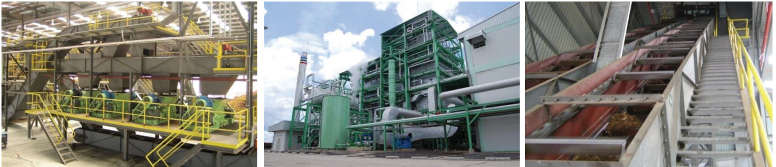
Figure 16: Photographs of biomass power plant in Malaysia, showing boiler house, fuel conveyor, EFB processing.
